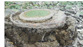
A corroded manhole in the Bay.
